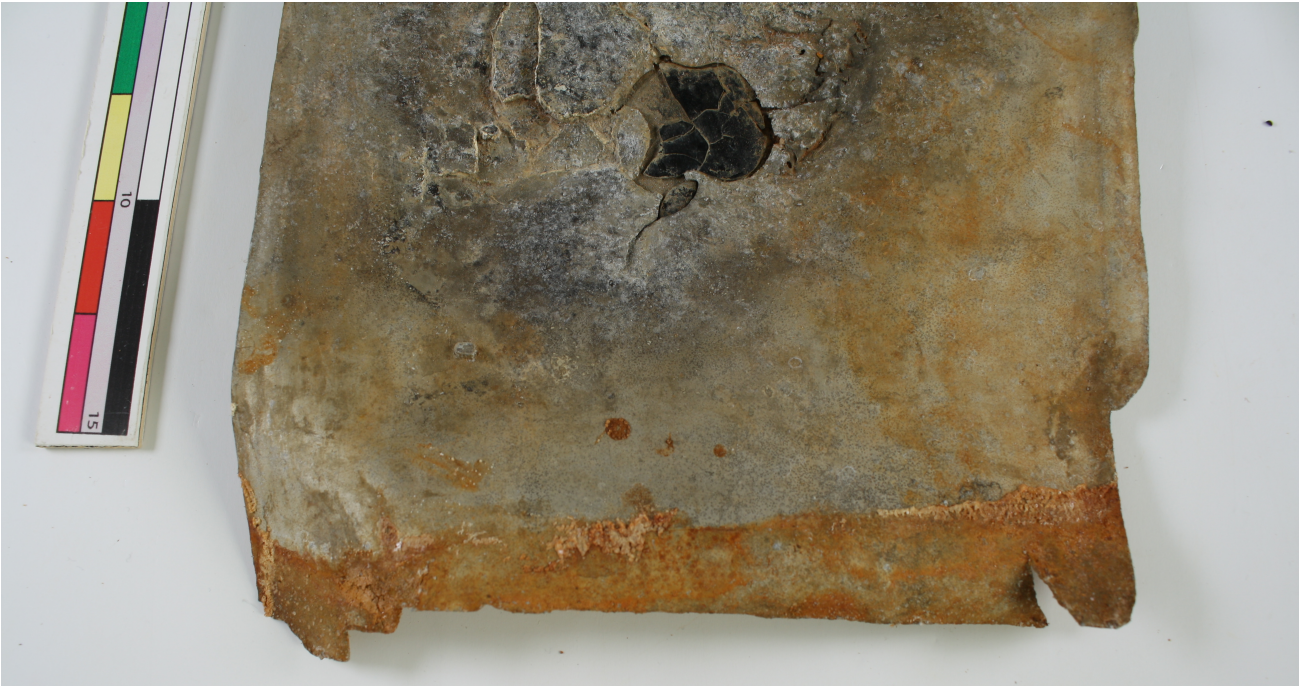
Image 6. The top edge on the front side, showing area of increased corrosion and jagged edge.
