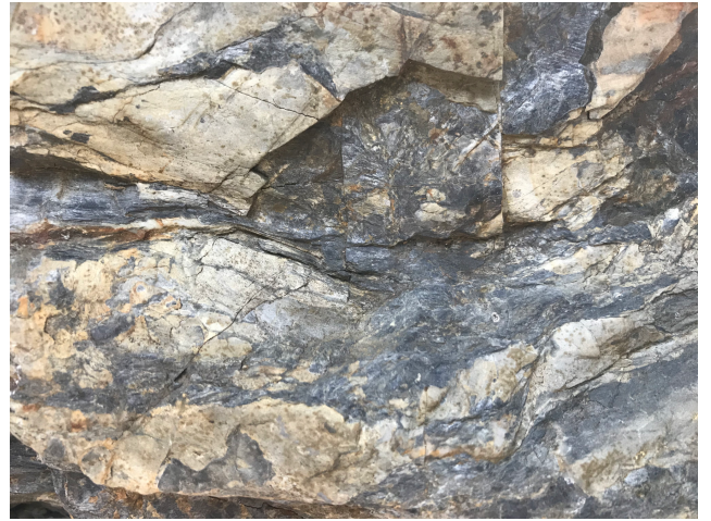
Fig.4 Fine straight hairline crack, sharp and straight breaking edges. Indicating the tendency to break into flat pieces
